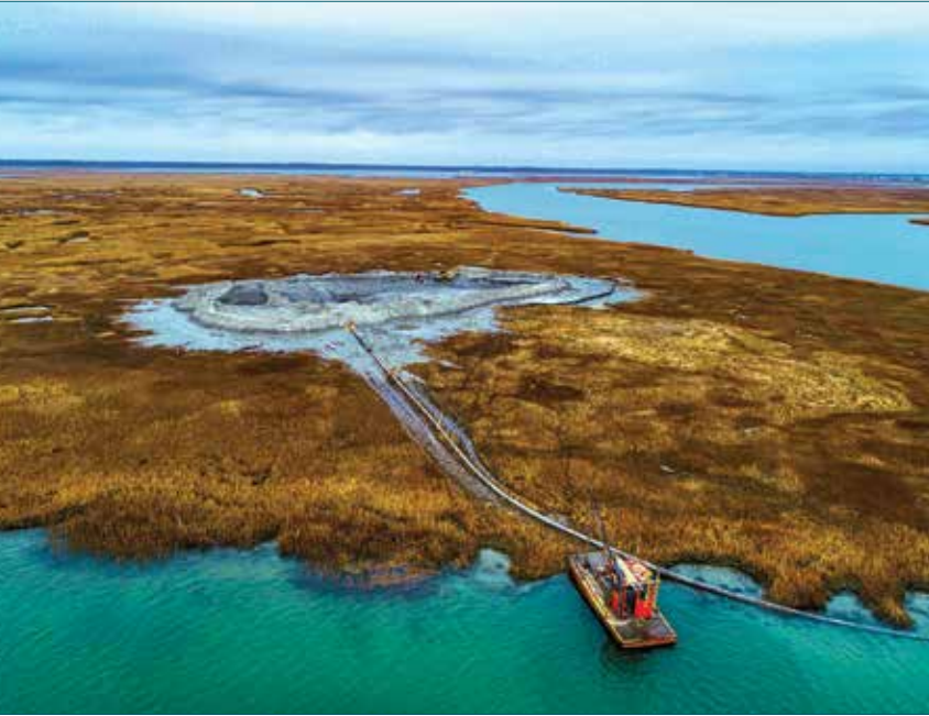
The U.S. Army Corps of Engineers and its contractor Barnegat Bay Dredging Company completed a dredging and marsh restoration project near Stone Harbor, N.J. in December 2018. Work involved dredging sediment from the channel of the New Jersey Intracoastal Waterway and beneficially using the material to create habitat on marshland owned by the New Jersey Division of Fish & Wildlife. Credit: USACE.
